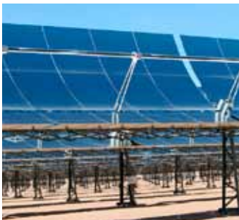
A solar farm.
